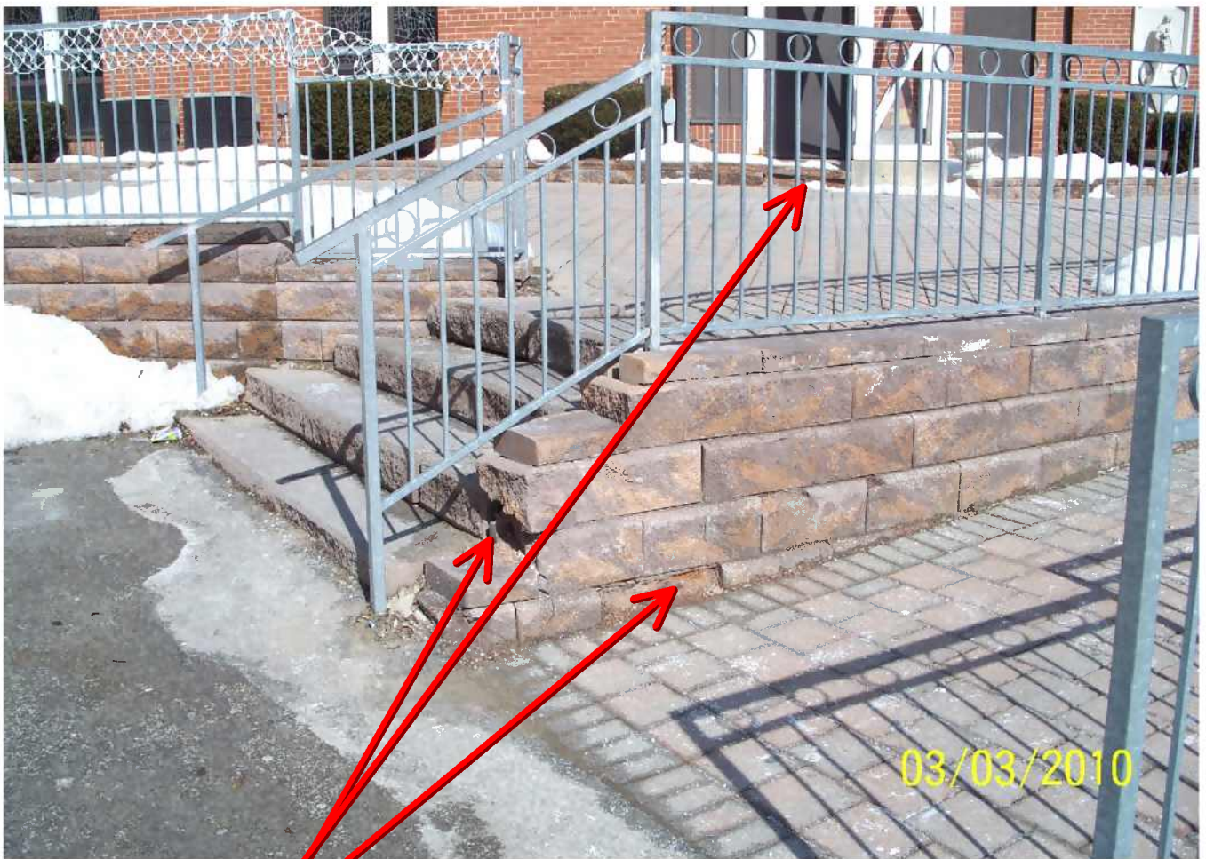
Photos showing more deterioration.
